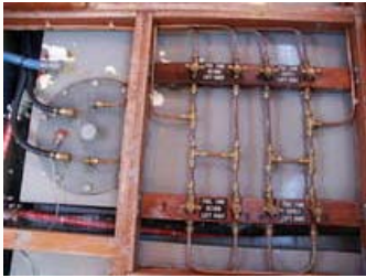
Fuel tank delivery system
