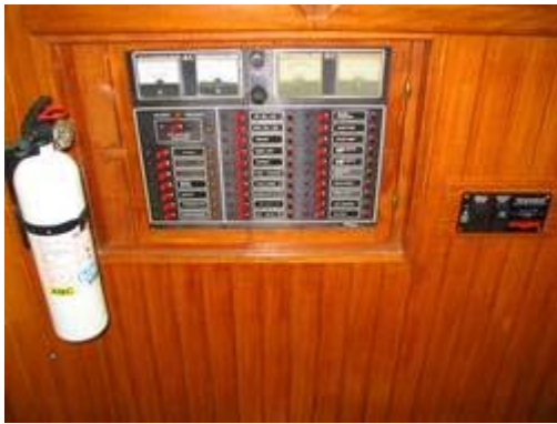
AC/DC Distribution Panel
